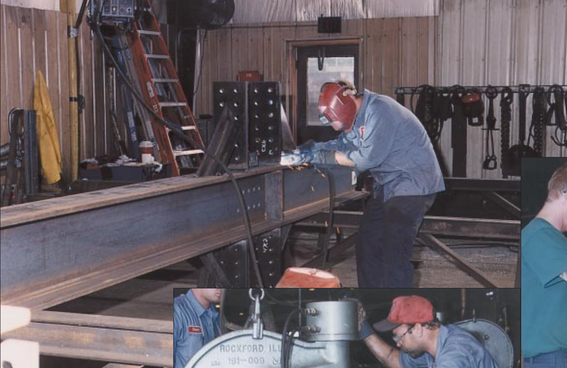
Welder in McFarlane's fitup area attaches beam seats to a structural column.
